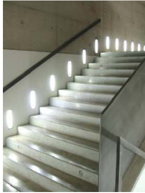
Fig. 6. Escape lighting for staircases.
